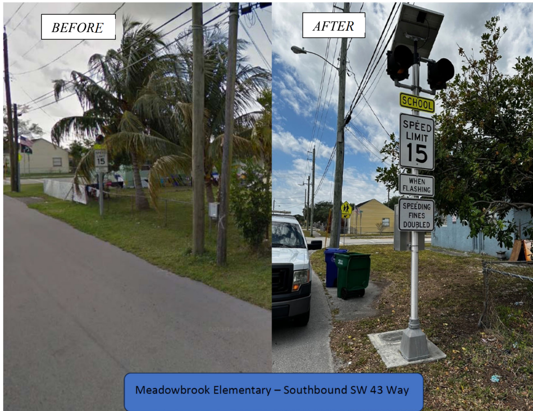
Figure 5: Example of Single-to-Dual Post-Mounted Flashing Beacon Conversion
